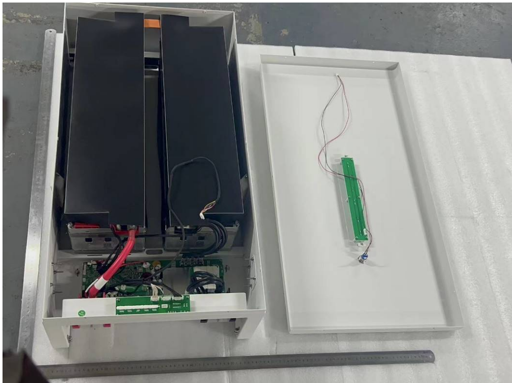
Internal View of battery module
